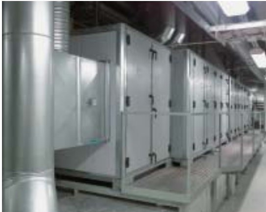
Air handling units (AHUs) of an office building.
